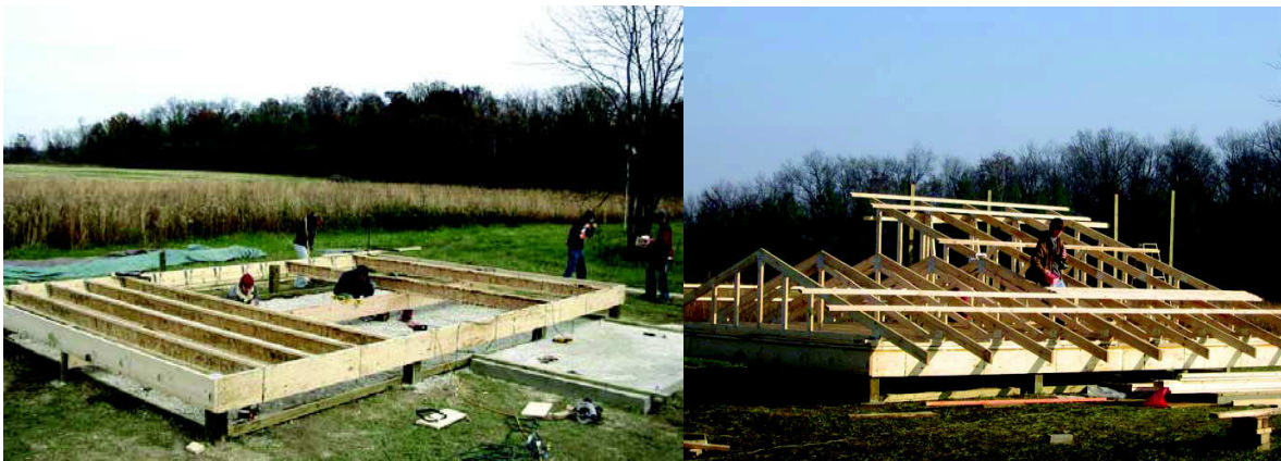
Figures 6, 7: Framing the platform with laminated veneer beams and truss joists, framing the roof trusses directly on the deck.
