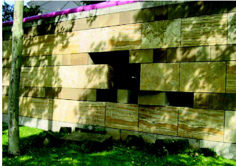
Figure 2: Solid blocks fall out of a rainscreen stone veneer. Neue Staatsgalerie, Stuttgart, Germany, 1988, James Stirling, Architect.
