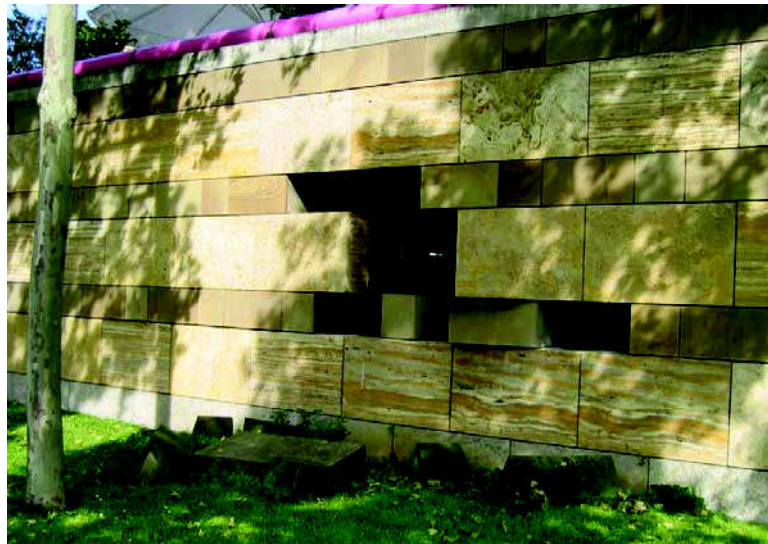
Figure 2: Solid blocks fall out of a rainscreen stone veneer. Neue Staatsgalerie, Stuttgart, Germany, 1988, James Stirling, Architect.
