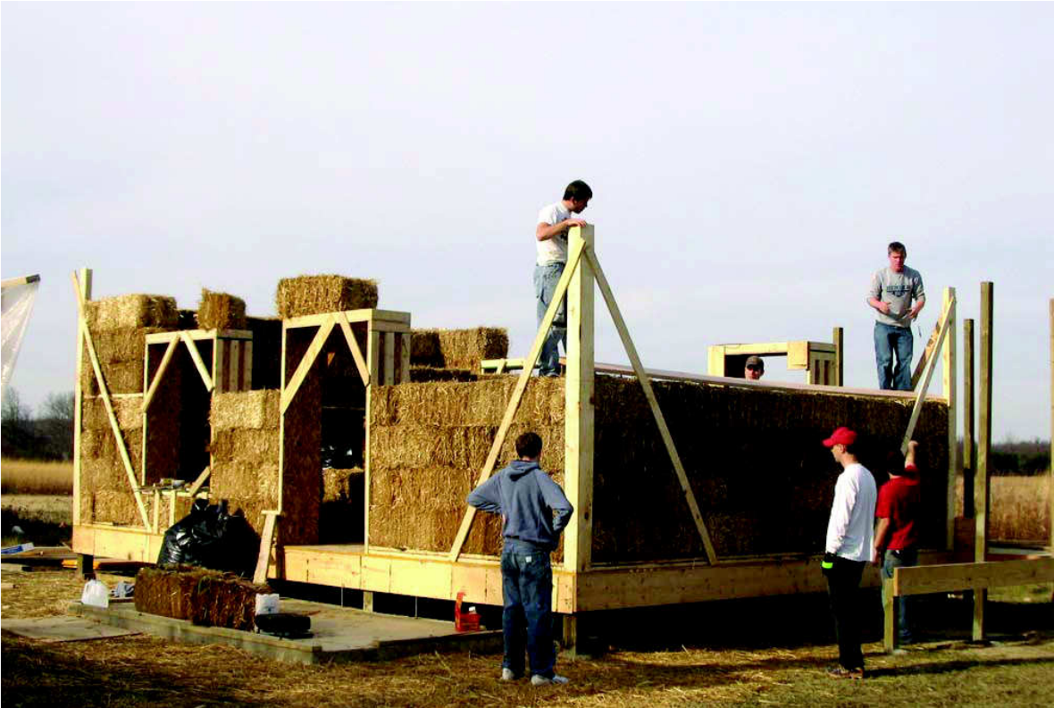
Figure 9: Installing 2x10 “beam” on the flat at the top of the fourth bale course to stabilize the wall horizontally.
