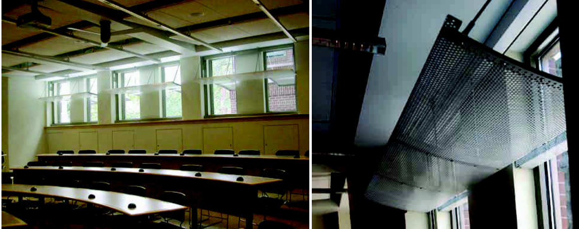
Figure 4: Light shelves and ceiling fans in a south-facing Lillis classroom (left photo courtesy of Emily J. Wright; right photo courtesy of SRG Partnership).
