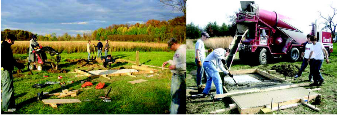
Figures 4, 5: Ground break in mid-October (at last!); pouring the slab and footings of the entry porch with fly-ash concrete
