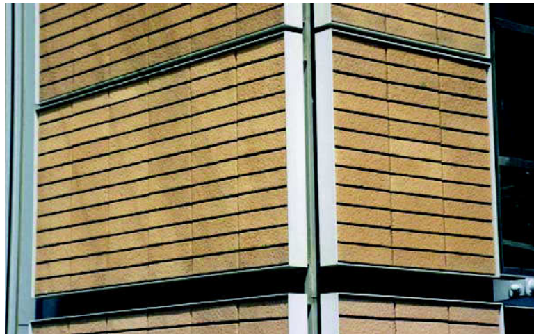
Figure 3: Cored bricks secured with plastic spacers on vertical rods. IRCAM, Paris, France, 1989. Renzo Piano Building Workshop.
