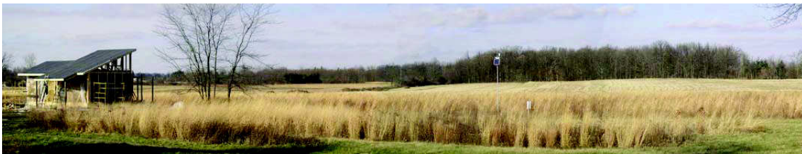
Figure 1: Eco-Center under construction sited at the south end of a restored prairie at the Cooper Field Station, Muncie, IN
