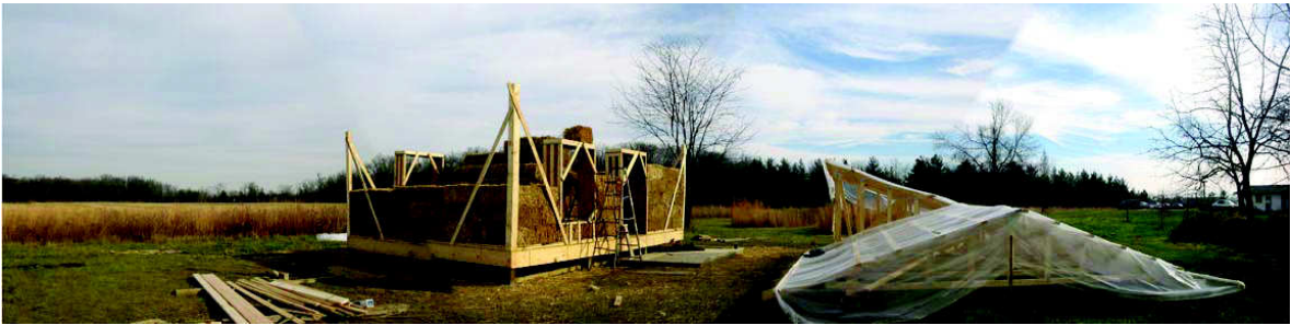
Figure 8: Erecting the bale walls; great lengths were taken to keep the materials dry through the course of construction.
