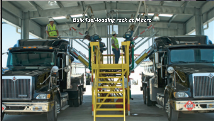
Eight fueling points help get emergency vehicles moving quickly
