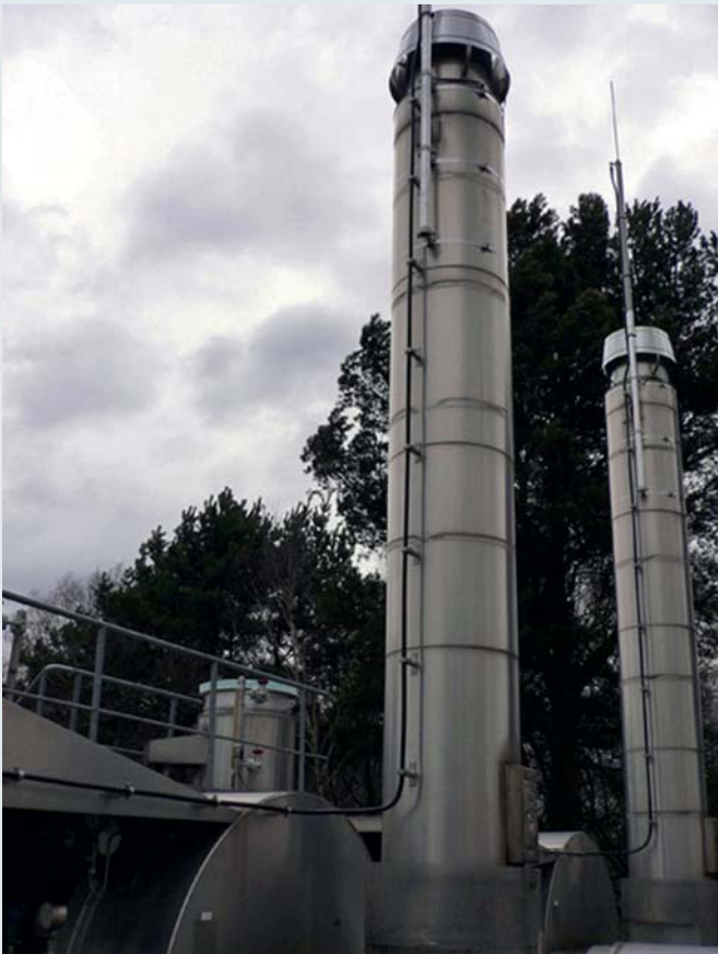
HVI conductor installed in Ex zone 2
