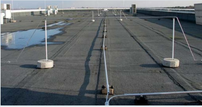
Elevated air-termination system with spacers and concrete bases in the range of the electrical installation on the roof
