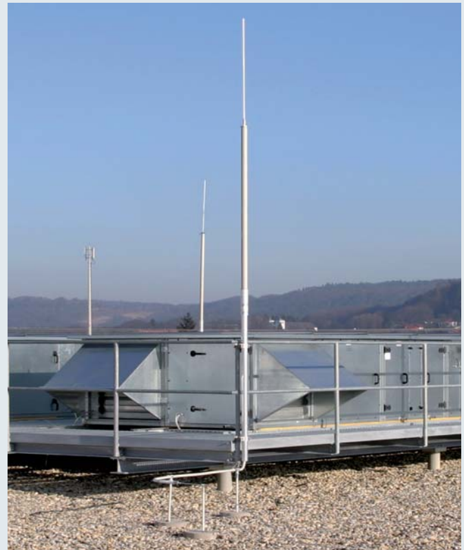
Isolated air-termination system for recooling plant with HVI conductor grey in a supporting tube
