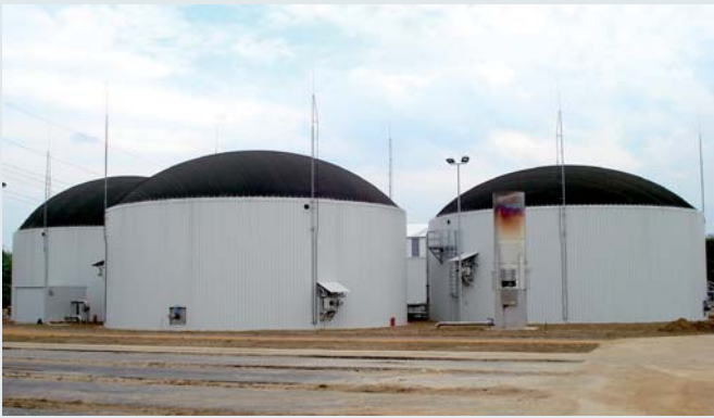
Biogas/natural gas plant Kerpen, Germany Protection of the fermenters – air-termination masts with HVI Conductors
