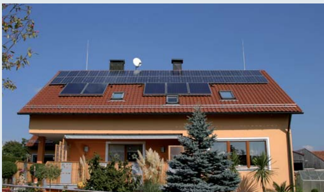
Isolated air-termination system – all roof-mounted structures such as solar thermal, PV and exhaust systems incl. the parabolic antenna in the protective area
