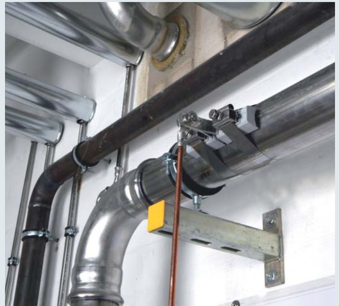
Installed on a StSt pipe
