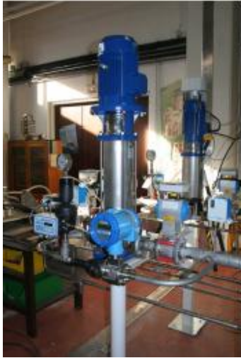
Figure 7: Cold water injection line
