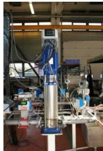
Figure 6: Hot water injection line
