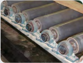
Overheating conveyor bearing
