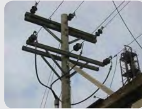
Distribution line faults
