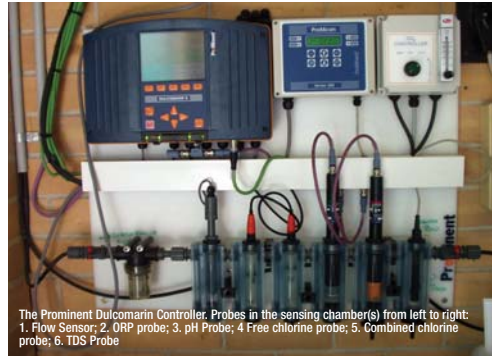
The Blue I controller showing the in-line photometer (door open) with three containers of reagents fed every five minutes into the testing chamber. (Kindly provided in monitoring mode only for the field day by Nubian Water Systems.)
