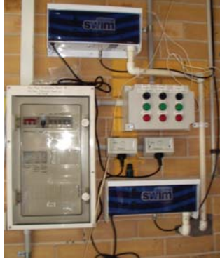
The two Ozone Swim generators
