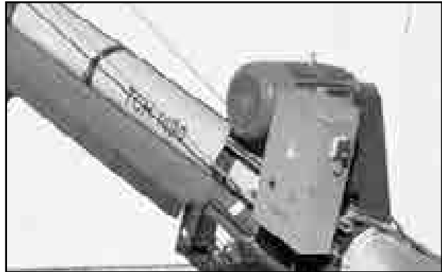
Fig 69 - Motor Control Box
