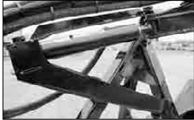
Fig 56 - Hydraulic Valve on Discharge Swing Lift Arm
