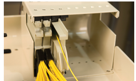
Feeder Pass-Thru Feature
