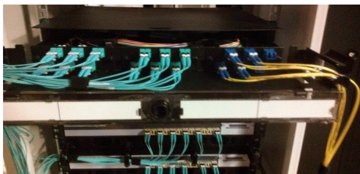
Figure 22: Fiber connections to FAPs inside of FRME1U. Yellow is for management ports. Aqua is for the Fiber Switches.
