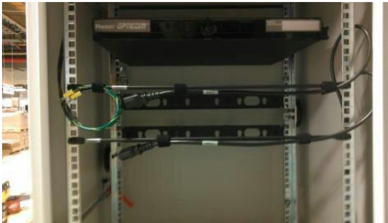
Figure 24: Horizontal support bar with ground cables and AC power cords.
