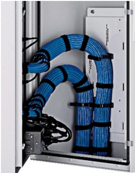
Figure 12: Copper Cable Routing showing Switch-A on the left and Switch-B cables on the right.
