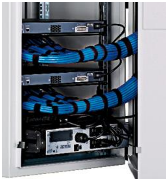
Figure 13: Switch-A (lower) and Switch-B (upper) copper cable bundles attached to strain relief bars.
