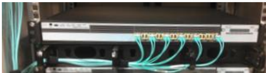
Figure 28: Fiber Switch A and B mounted to front rail showing fiber cable routing.
