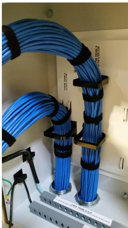
Figure 20: Copper Cable Routing showing Switch-A on the left and Switch-B cables on the right.
