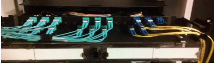
Figure 29: Fiber connections to FAPs inside of FRME1U. Yellow is for management ports. Aqua is for the Fiber Switches.
