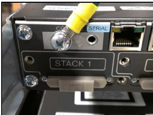
Figure 31: Ground cable connection to the Fiber switch.
