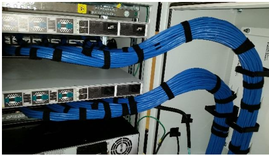
Figure 22: Switch-A (lower) and Switch-B (upper) copper cable bundles attached to the rear strain relief bars.
