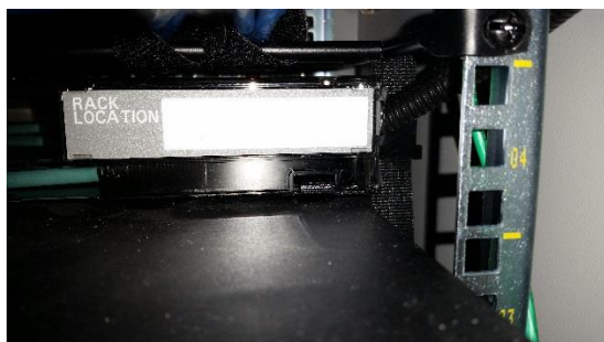
Figure 17: Loom tubing routed around hinge point and rail.
