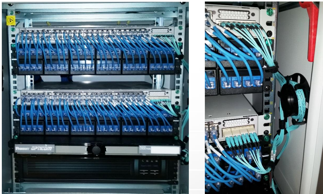
Figure 25: Switch-A (lower) and Switch-B (upper) switches showing fully populated patch cords.
