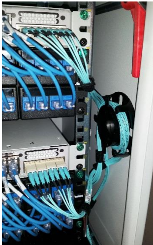
Figure 30: Fiber Patch Cord Slack Management
