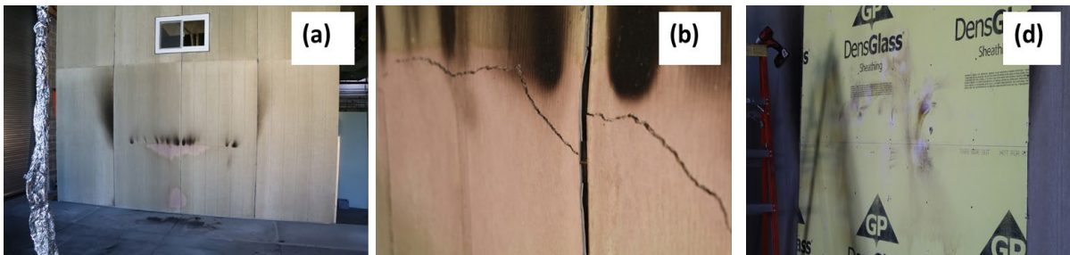
Fig. 86. Photographs of target structure showing (a) overall marginal damage to the exterior wall, (b) some cracking of cement board, and (c) some discoloration of DensGlass® seen after removal of cement board in test 1B-SCI0-0.
