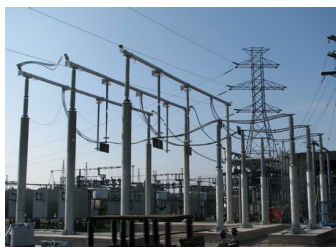
FULL SCALE SHORT CIRCUIT TESTING TO 63 kA/1sec POWERTECH LABORATORY, VANCOUVER, 2009.
