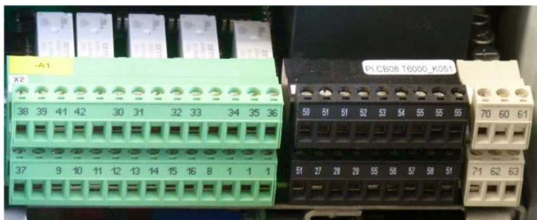
Figure 8-13 Control cable terminals
