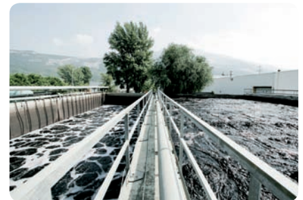
The water treatment plant in Rovereto (Trento).
