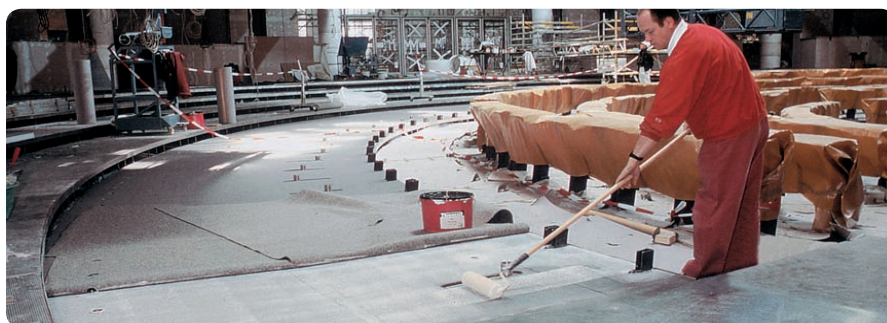
Headquarters of the German Parliament (Berlin): textile flooring made with Alto Chroma Aquafil yarn.
