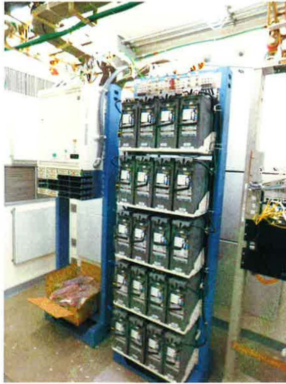
Photo 5: Sample photo illustrating the existing equipment.
