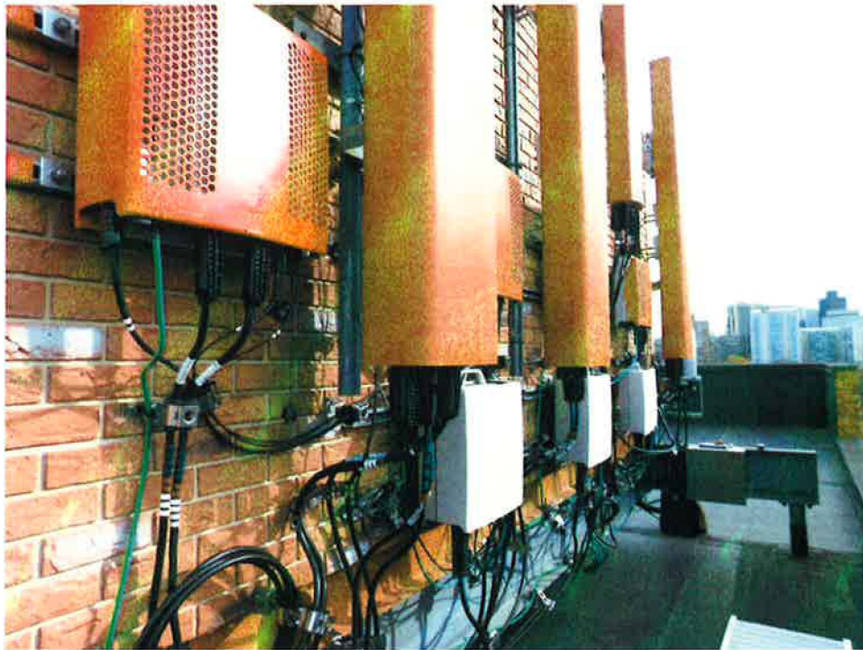
Photo 3: Sample photo illustrating the existing Gamma sector antennas and RRH's.
