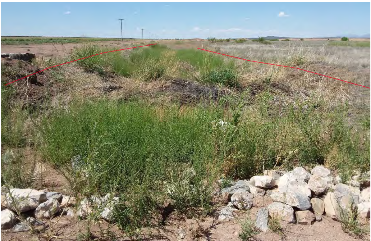
Figure 62 Photo Point U1, looking upstream into the U.S. Again, water is ponded by road crossing. Appears to be fed by field tailwater.
