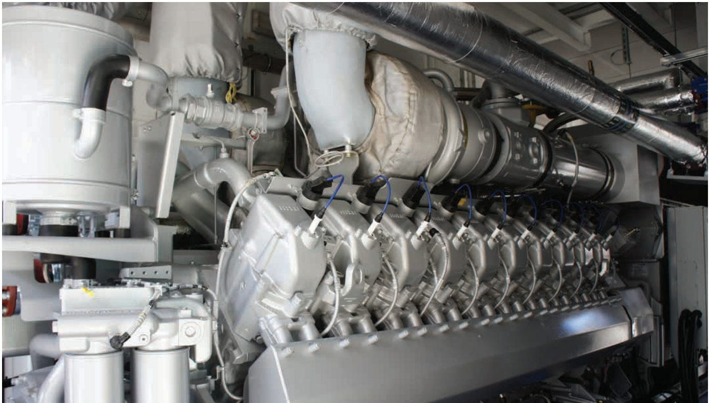
Combined heat and power units at Bunhill and Dalston
