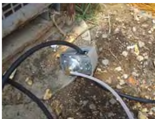
Fig. 3. A view of the pressure switch at the Horticulture Services Building (Macdonald Campus, Sainte-Anne-de-Bellevue, QC, Canada) that turns the 1-horsepower (0.75 kW) centrifugal water pump on and off for irrigation, when the line pressures are 25 and 40 psi (172.4 and 275.8 kPa), respectively.
