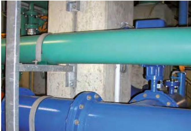
Pipe supports on vertical HZA Channels
