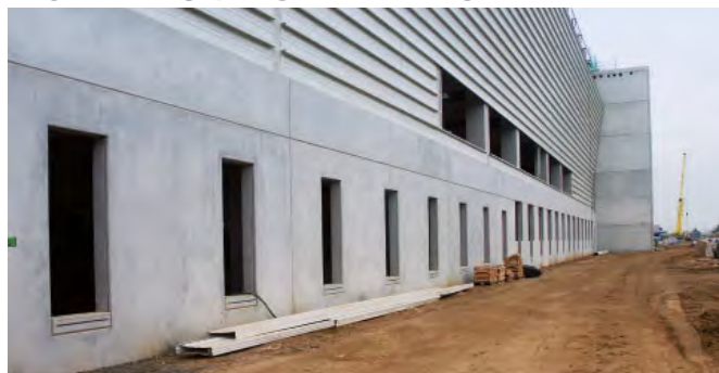
UPS Air Hub, Cologne Bonn Airport, Germany
