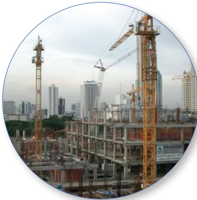
Noise Emission Monitoring
