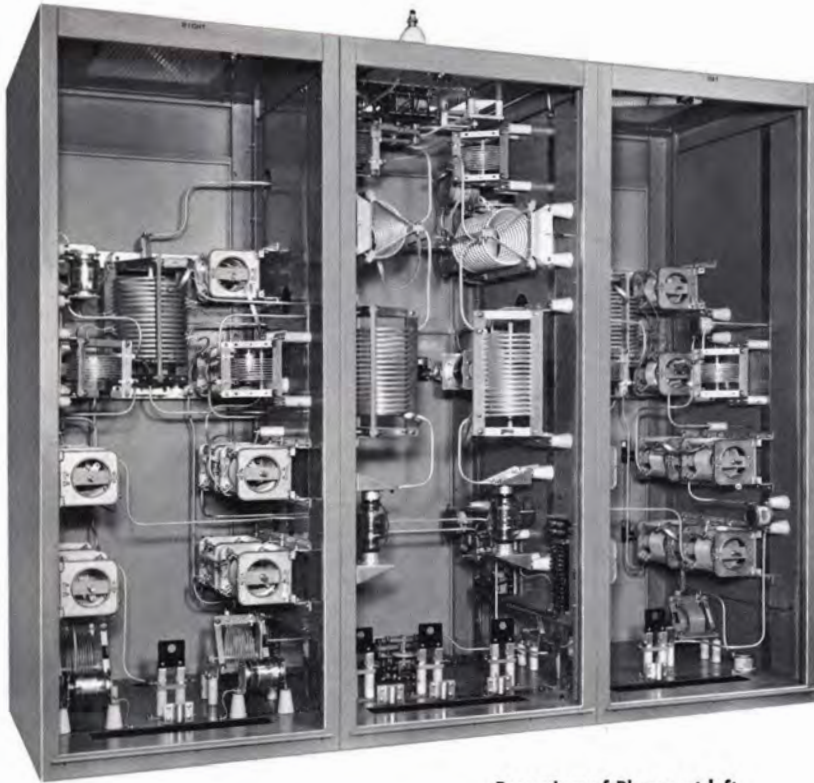
Rear view of Phasor at left, with panels removed. Note the clean mechanical layout.
