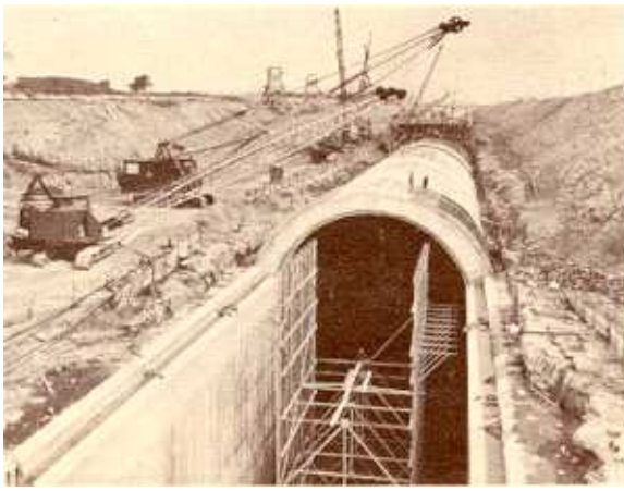
Conduit #1 Niagara Power Project under construction, September 1959—Power Authority—State of New York.
