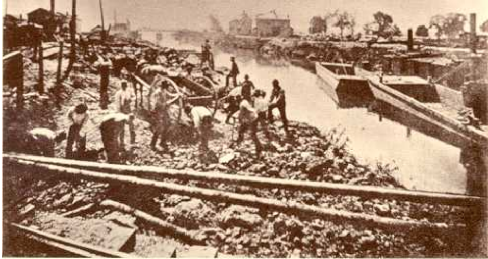
Widening the Hydraulic Canal across the City of Niagara Falls was no easy job in the 1890's.
