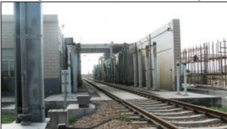
Figure 20.1 CRH EMU Car Wash Facility
