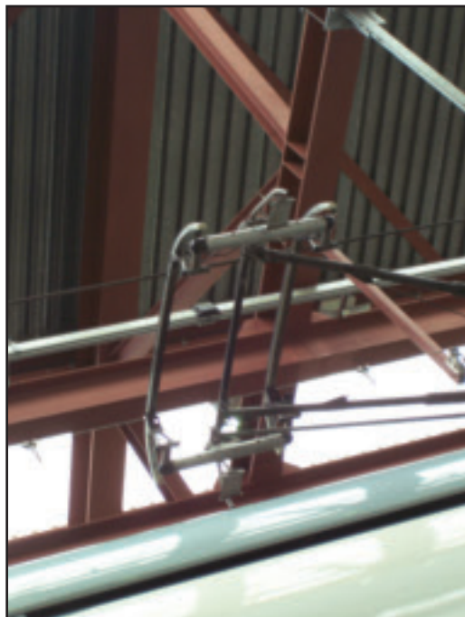
Figure 16.4 Velaro E Pantograph Interface with Contact Rail at NERTUS Facility
