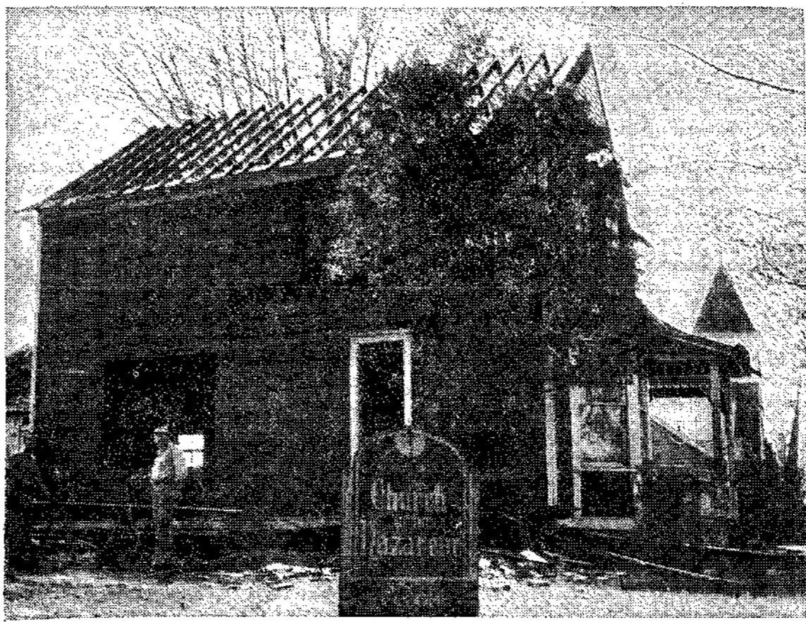
"WELCOME"—says the sign, but if you're planning on staying, you'd better bring your umbrella because there's no roof on the Nazarene Parsonage. The 75-year-old building is being torn down to make way for a $17,000 one-story, three-bedroom home. Work on the new parsonage is being done mainly by Rev. Richard Spencer and Lawrence Cox and other church members. (Chronicle photo)
