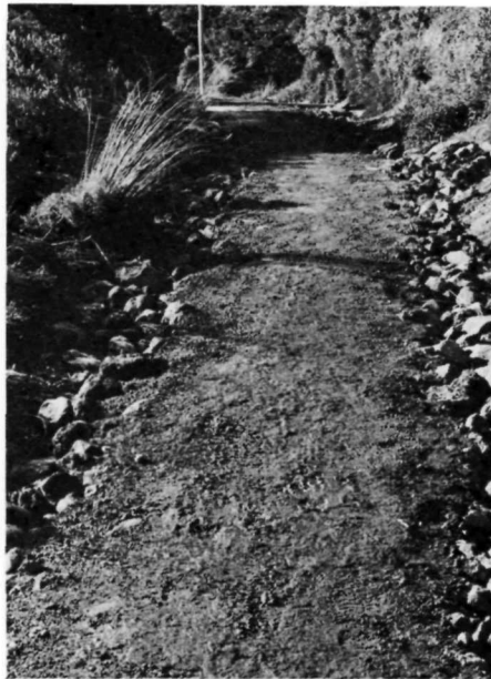
The same area as shown at left after treatment. In this particular case boulders were used to fill in eroded sections and to provide a good drainage base. A layer of fine angular gravel was then applied as the walking pad. Replanting was done where the track had been unduly widened by walkers avoiding the wet and eroded sections.
