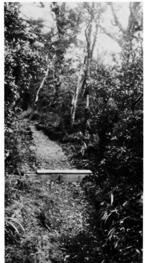
Surfacing the track is often necessary. Angular-shaped gravels offer the best binding qualities. Roundish gravels “move” with the constant walking action and will eventually disappear from the walking surface. Watertables and culverts must be incorporated at intervals sufficient to disperse the surface run-off.
