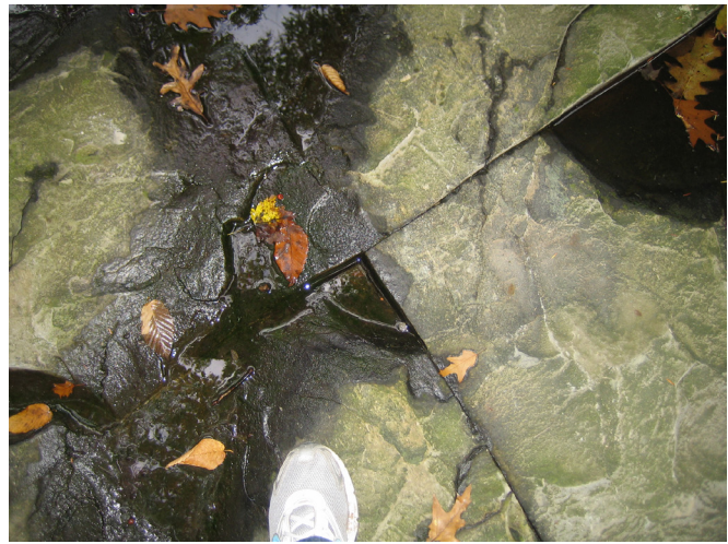
Figure 20. Photograph of jointed bedrock near Mary Campbells Cave. Through-going joints and fractures provide conduits for trickling groundwater as well as provide planes of weakness that preferentially weather and may break when the stress is applied to the bedrock. Photograph by Trista L. Thornberry-Ehrlich (Colorado State University) taken in autumn 2009.
