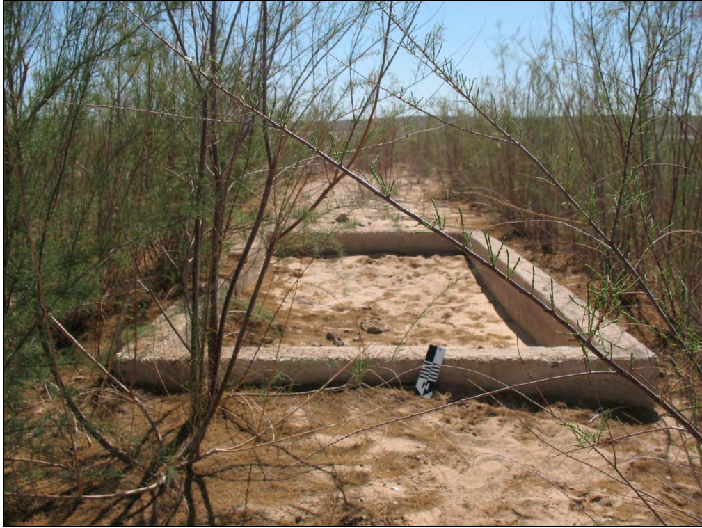
Figure 33. Tamarisk is one of the many invasive plant species that threaten not only the native ecology but also cultural resources within the park. Tamarisk has had a heavy impact on the historic town site of St. Thomas, as seen in this picture of a structure foundation. Courtesy of the National Park Service.
