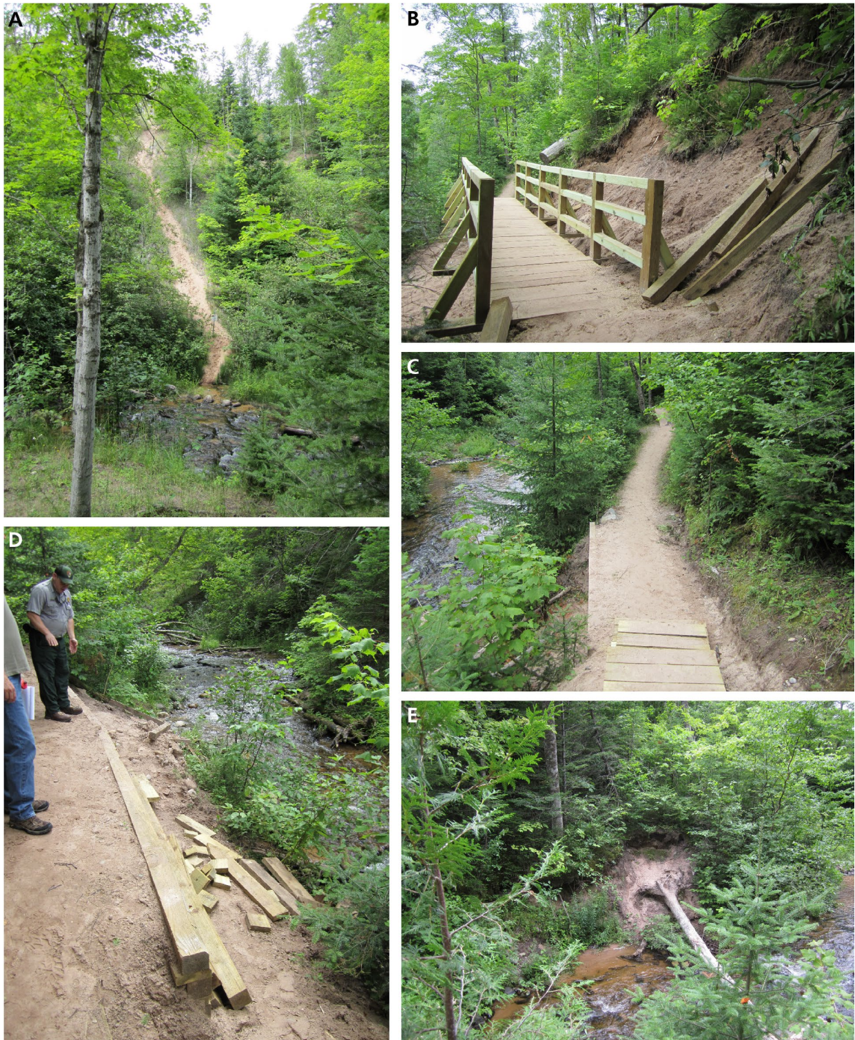
Figure 29. Photographs of trail rehabilitation projects and a social trail up the side of a dune. (A) Social trail use has created an unstable (de-vegetated) slope along the side of an active dune. The lakeshore staff have attempted to use signage to discourage access. (B, C, and D) The trail down to the base of the Grand Sable banks along Sable Creek was the subject of significant restoration work as erosion, stream channel migration, and overuse threatened several stretches. (E) Natural stream meandering and erosion causes treefall along stretches of lakeshore streams. This can expose more sediment to the adjacent stream channel. Photographs by Trista L. Thornberry-Ehrlich (Colorado State University) taken in summer 2009.
