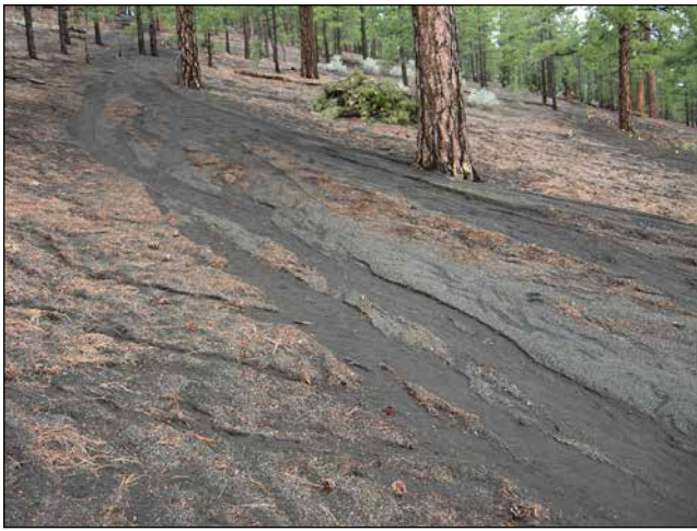
Figure 4.5.4-3. Trail ascending Lenox Crater was washed out by heavy rains in 2016. Photo Credit: NPS/P. Whitefield.
