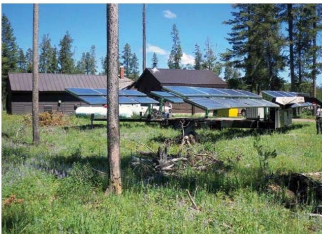
This portable photovoltaic system at Bechler provides power during the summer season, meeting 90% of the site's electrical needs.
