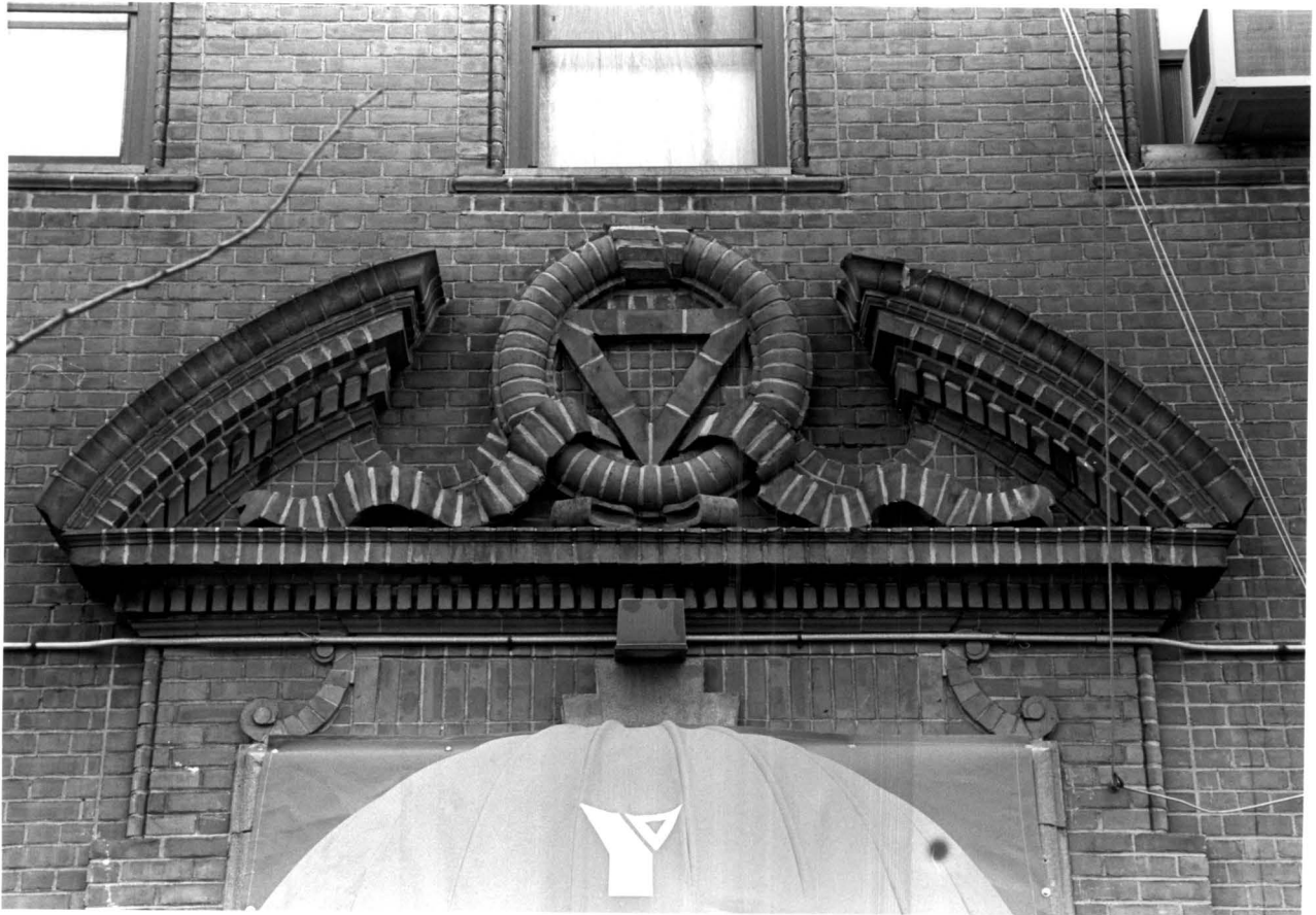
Young Men's Christian Association (YMCA) Building, 135th Street (later Harlem) Branch Entrance details Photo: Carl Forster
