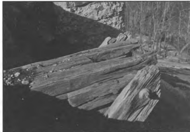
DURING the REMOVAL PROCESS, the ENCASED TIMBERS by the south trestle abutment are exposed. (1994 photo by Judi Schroeder)
