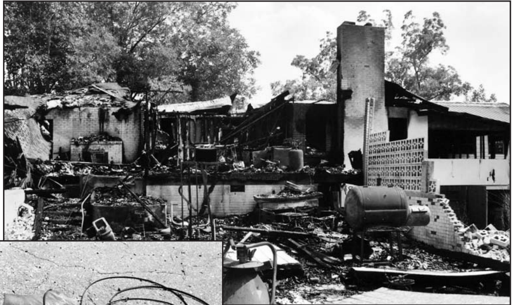
Residence was destroyed by Fire and BLEVE.
