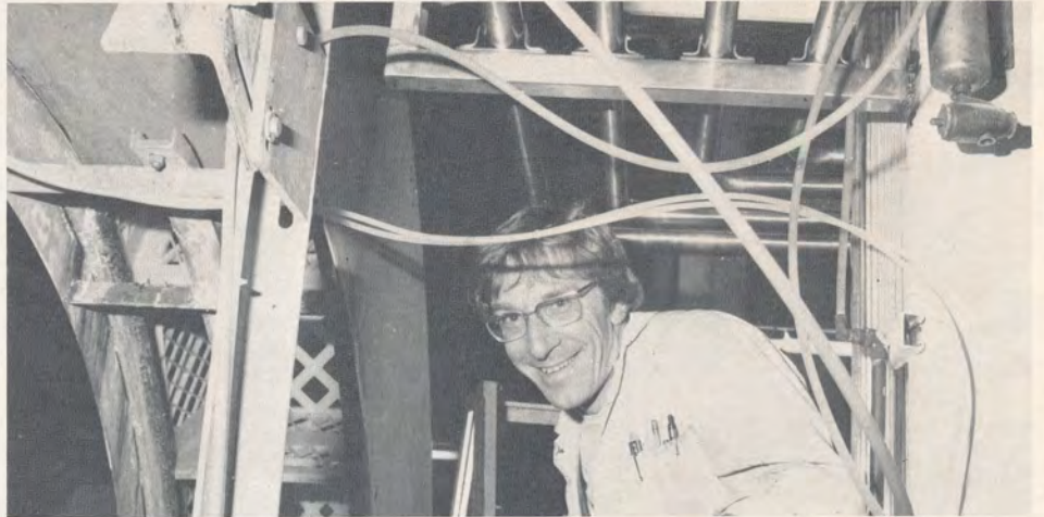
The piping above Al Wheatley will provide cleaning water to all fluid-line machines.
