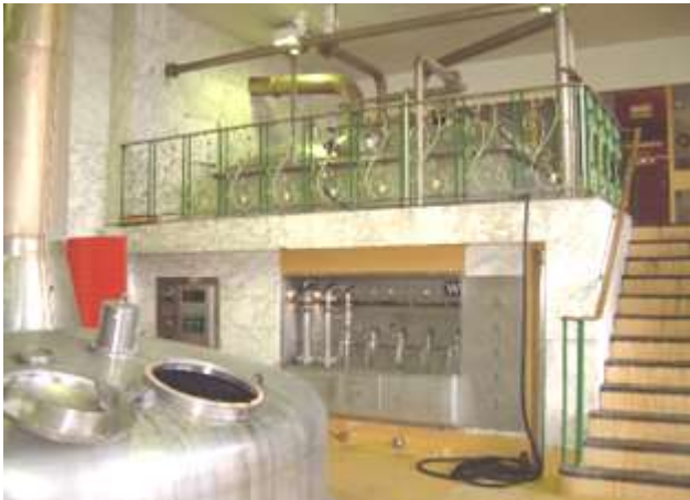
The Strainmaster is on the mezzanine level above the wort inspection station. The copper is in the foreground
