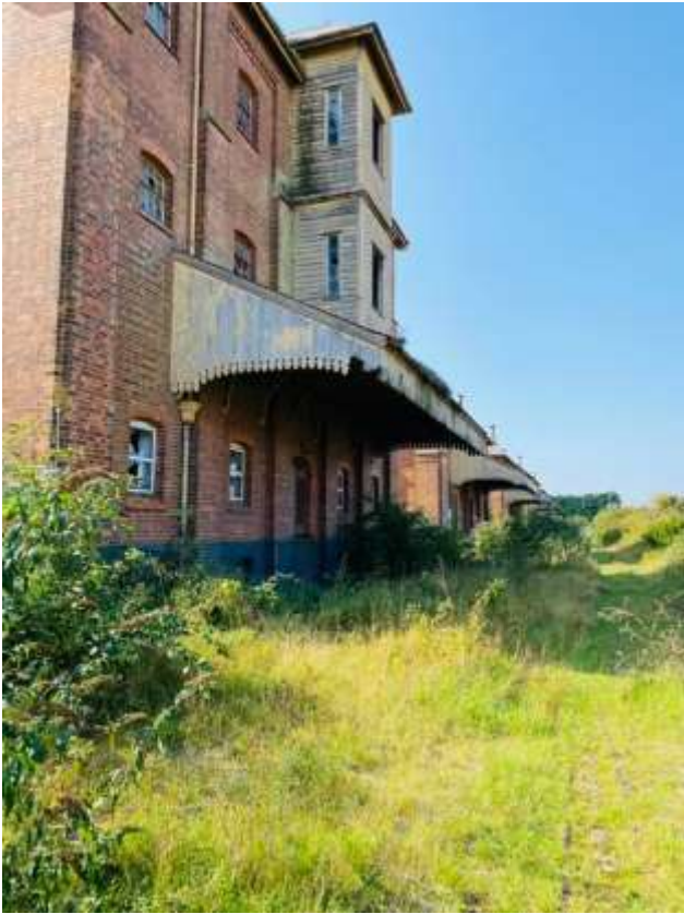
The Bass maltings complex at Sleaford has been empty and unloved for over twenty years.
