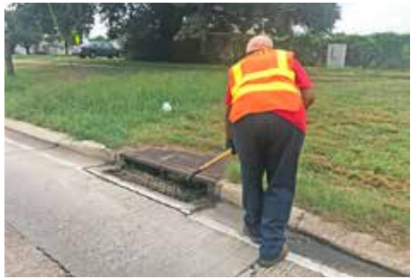
A DOTD worker clearing debris from a storm drain in Bossier Parish in preparation for Hurricane Harvey in 2017.
