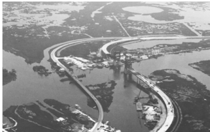
Old LA 1 bridges in Leeville in 1969. The vertical lift bridge on the right is under construction.
