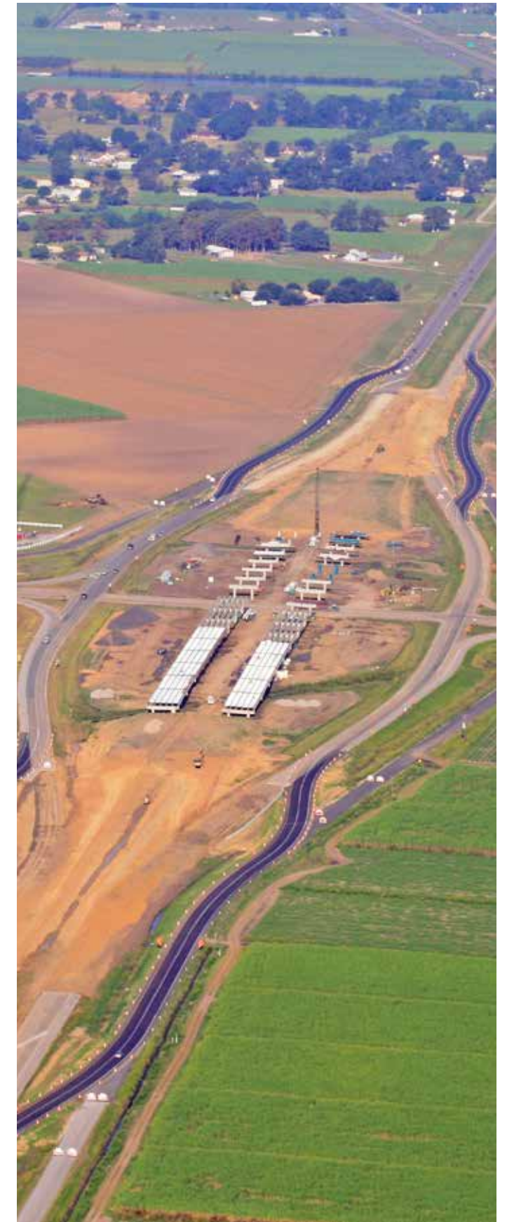
This U.S. 90 interchange with LA 85, shown ca. 2010, will eventually become an I-49/LA 85 interchange.
