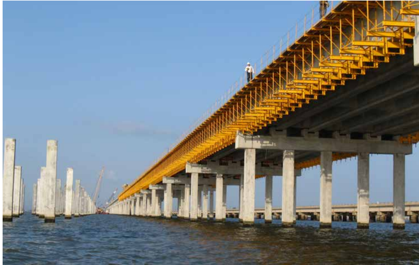
I-10 Twin Span Bridge between New Orleans and Slidell being reconstructed after 2005's Hurricane Katrina.
