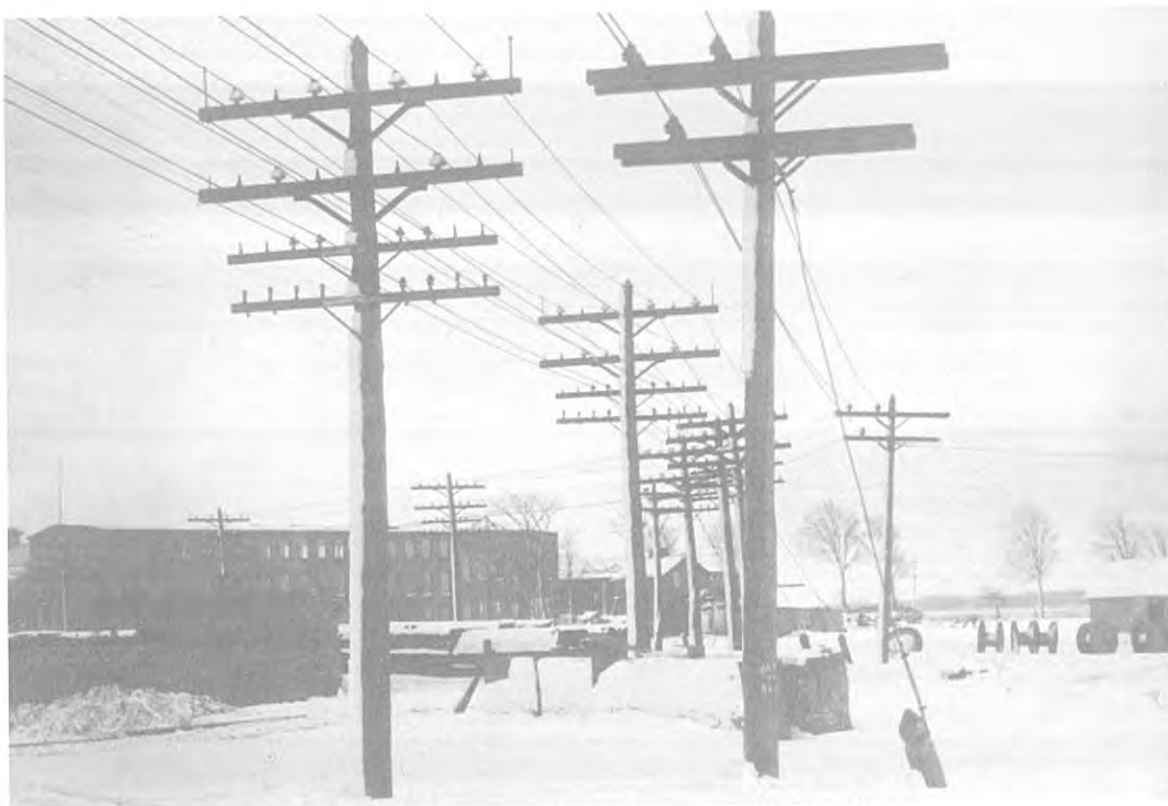
10,000 volt transmission line at Niagara Falls, New York.
