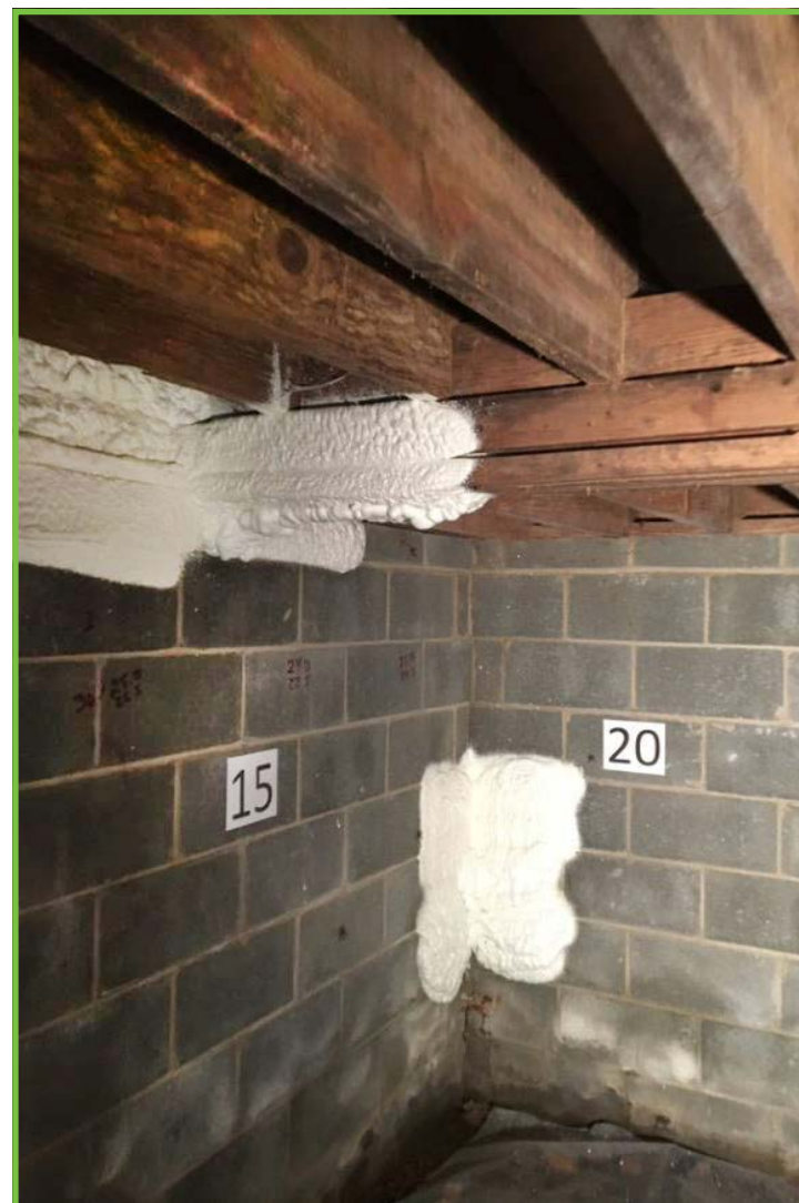
Spray foam insulation applied strategically in a crawl space beneath UGA's River Basin Center in Athens allowed pest control inspectors to test the latest technology for finding subterranean termites. (Derrick Lastinger/GDA)
