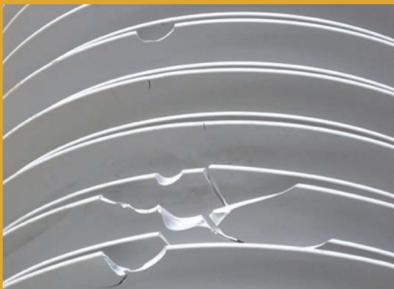
Damage to 800 kV bushing used at European-based test laboratory.
