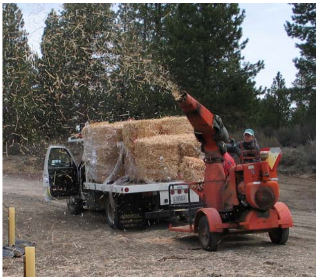
Figure 10.1.3.11. Straw blowers range in size from machines which can apply 30 to 60 bales per hour (shown here) to very large straw blowers that can shoot up to 20 tons per hour.
