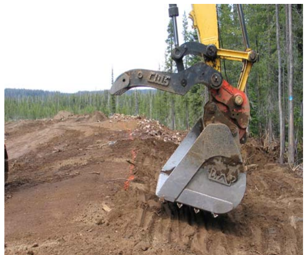
Figure 10.1.2.6. An alternative form of imprinting road cuts and fills that does not compact soils is welding angle iron onto the bucket of an excavator. As the excavator pulls topsoil into place and contours the slope, it presses the face of the bucket into the soil surface to form surface imprints.
