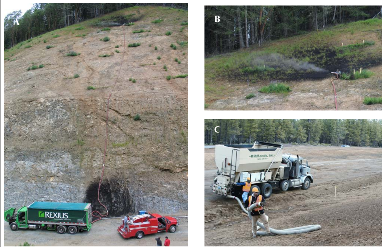
Figure 10.1.3.8. Wood fiber mulch is applied on steeper slopes with mulch blowing equipment. Large trucks can hold between 75 and 100 yards of mulch (A) while smaller trucks can hold up to 25 yards (C). Mulch is pneumatically delivered to the site through an application hose which can reach several hundred feet up steep slopes (A) with still enough force for ample delivery of mulch (B).
