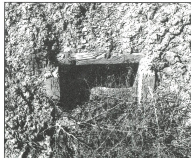
Wooden box culvert of type used on Salt Lake Wagon Road between Westwater and Grand Junction in later days.
