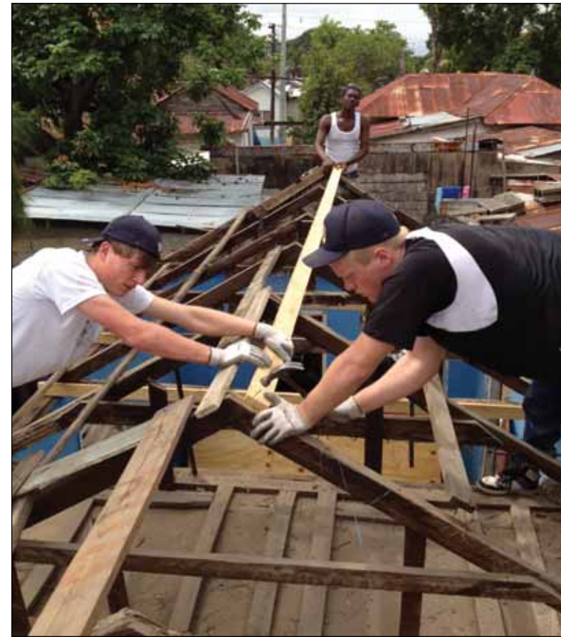
SAS juniors Alex Tinsley (left) and Russell Mays repair a roof in Whitfield Town.
