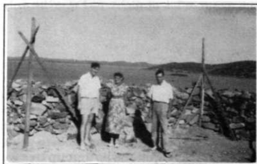
Left: Progress, as the walls rise higher. A view of the glorious setting of the new Church
