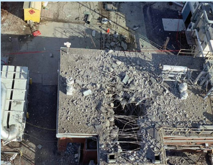
A section of the roof on the Deep Depth Test Facility in Building 179 blew out after an explosion on Feb. 24, 1995. (Photo published in April 1995 'NUWScope')
