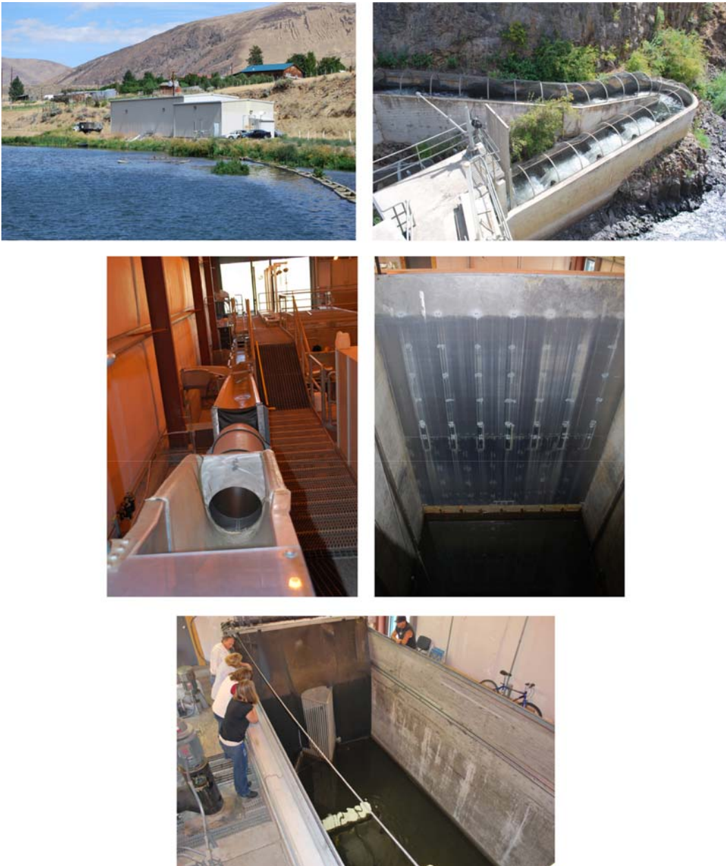
Figure 2-3. View of exterior of Roza adult fish collection facility (top left); pool and weir-type fish ladder (top right); fish chute to work area or back to river (middle left); fish lock (middle right); and adult holding tank (bottom, right).
