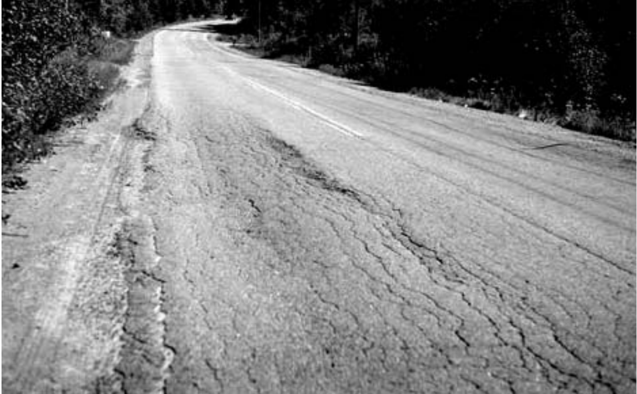
Figure 3-3: Base and Sub-Base Deficiencies
