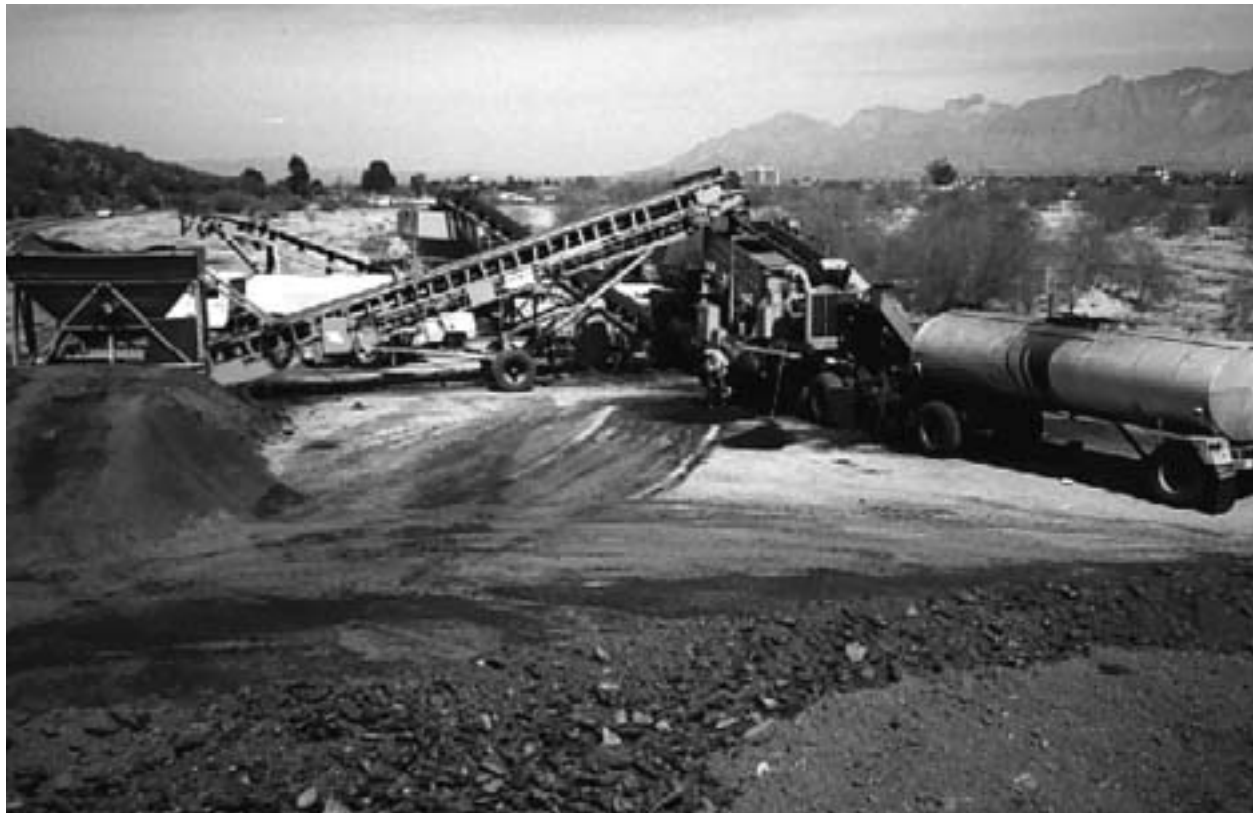
Figure 1-23: CIR train set up as a stationary plant
