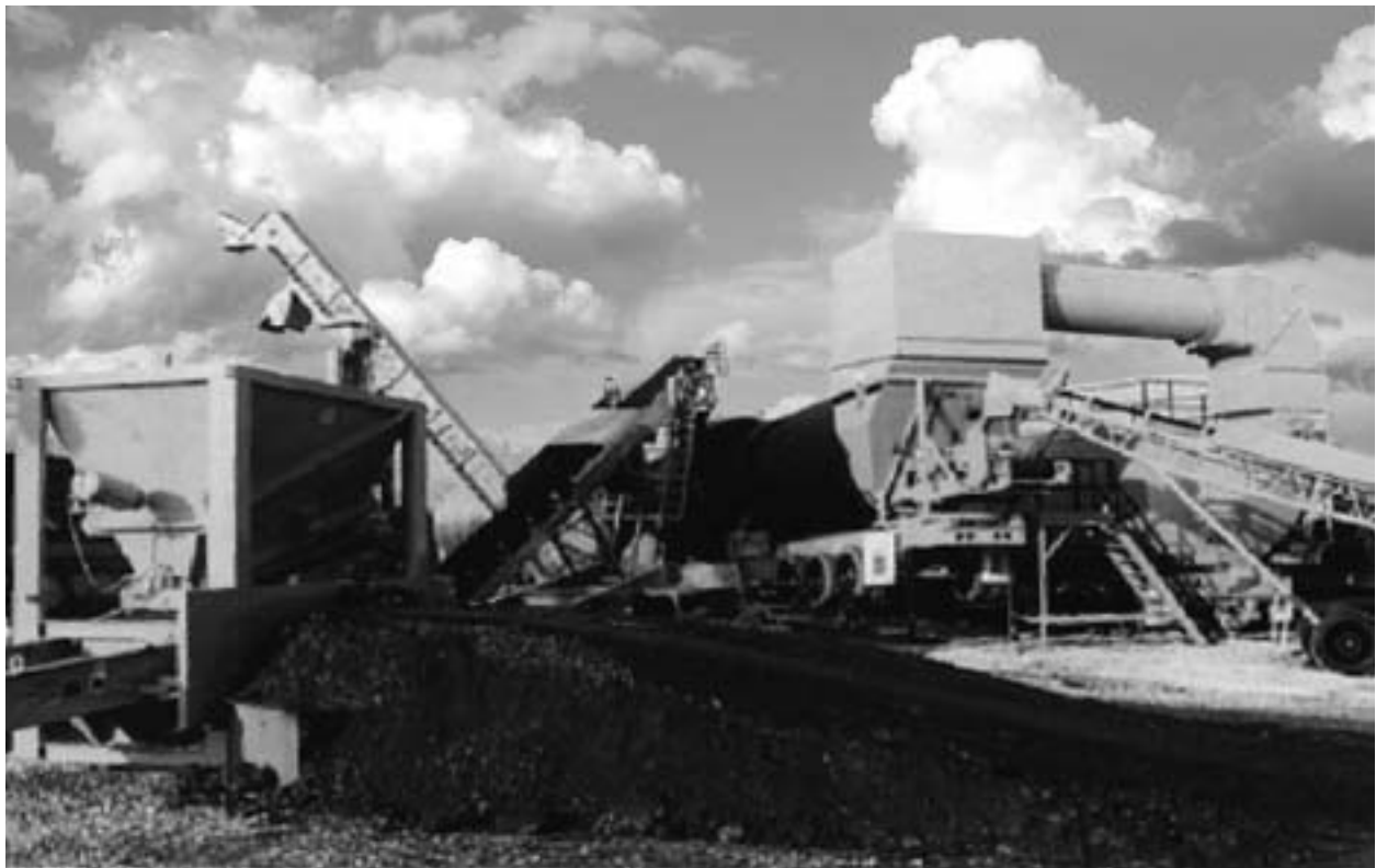
Figure 1-6: Drum mix plant with RAP infeed for hot recycling
