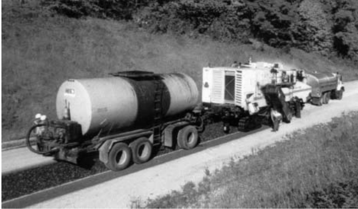
Figure 17-4: Connected Water (Front) and Emulsion (Rear) Tanks to permit Metered Addition of Both Liquids
