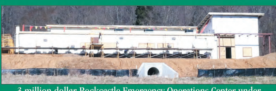
3 million dollar Rockcastle Emergency Operations Center under construction and completely paid for by Federal Government
