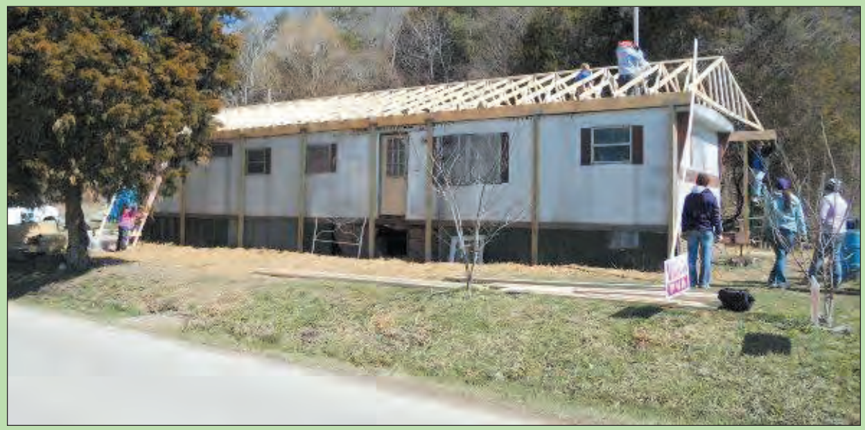
Around 100 college students from 17 different colleges have spent their spring breaks during the month of March making repairs to four homes in Rockcastle County. The students were participating in Christian Appalachian Project's Workfest program, which was created to help needy homeowners make repairs to their homes. The photo above is of a home being repaired in Wildie. Student volunteers built a new roof, a front and back porch, installed new windows and made several other repairs to the home. For more information about the program, contact CAP Housing at 606-256-0406. To qualify for repairs, participants must meet certain income requirements and own their own home.
