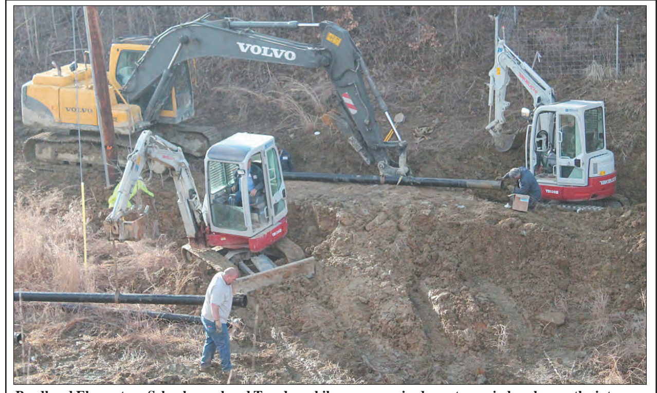
Brodhead Elementary School was closed Tuesday while crews repaired a water main break near the intersection of Chickadee Lane and Hwy 150 in Brodhead. City workers discovered the break Sunday afternoon during routine checks. The break wasn't repaired until Tuesday afternoon because crews had to order special parts from Tennessee. Brodhead water customers and businesses in Brodhead were asked to conserve water during the water main break because of the low water levels in the city's water tank. Brodhead water customers are still under a boil water advisory.
