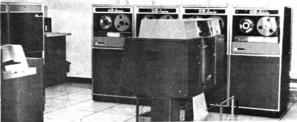
FB INSURANCE RECENTLY INSTALLED high-speed data processing equipment to continue its competitive position in the insurance world. The new electronic equipment, capable of reading and writing 22,500 characters per second on magnetic tape, is involved in all functions of the company's accounting and record keeping systems.
