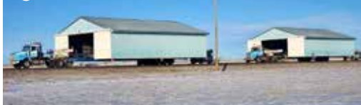
Two airplane hangers moved for Canard Shaw (Pioneer Acres). Canard was a building mover that retired many years ago.
