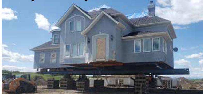
This 46x70, 3000 square foot home that we rescued out of the High River flood mitigation area.
