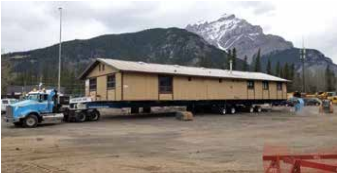
Canadian Pacific Railroad bunk house was moved from one side of the tracks to the other.
