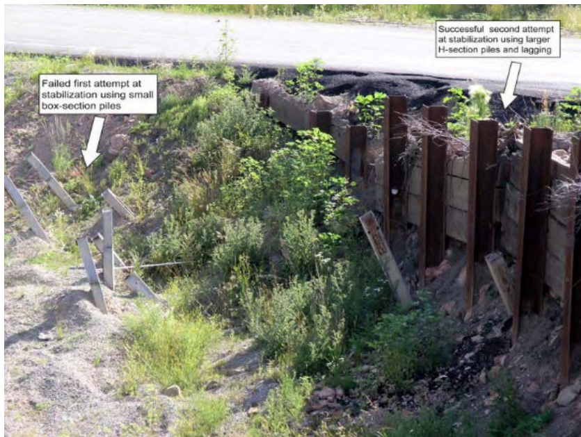
Failure and (at least temporary) success of driven piles to hold up Colorado Rt. 139, south of Douglas Pass (Kiousis et al., 2010).
